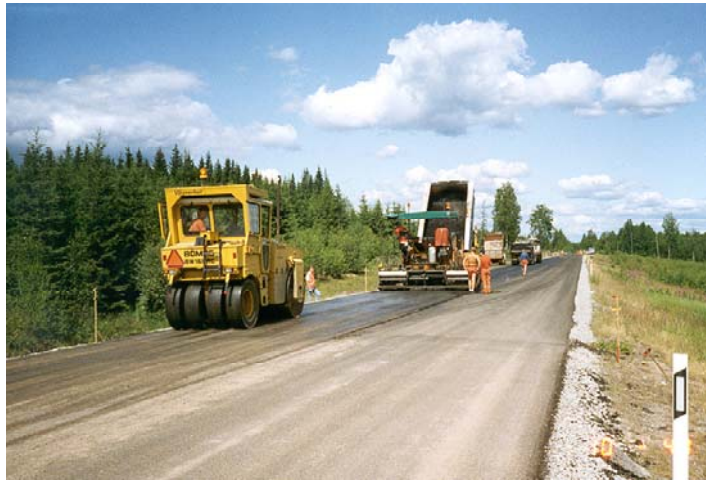
Figure 6 Laying and compaction of a cold recycled road base. In this case, a combined steel roller and rubber tyred roller was used.
