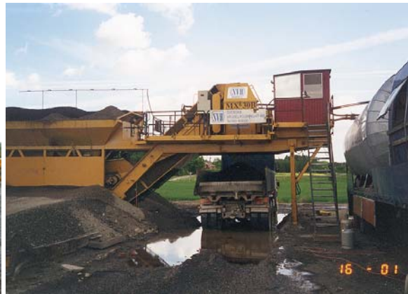
Figure 4 Mixing plant for batch production of cold mix.
