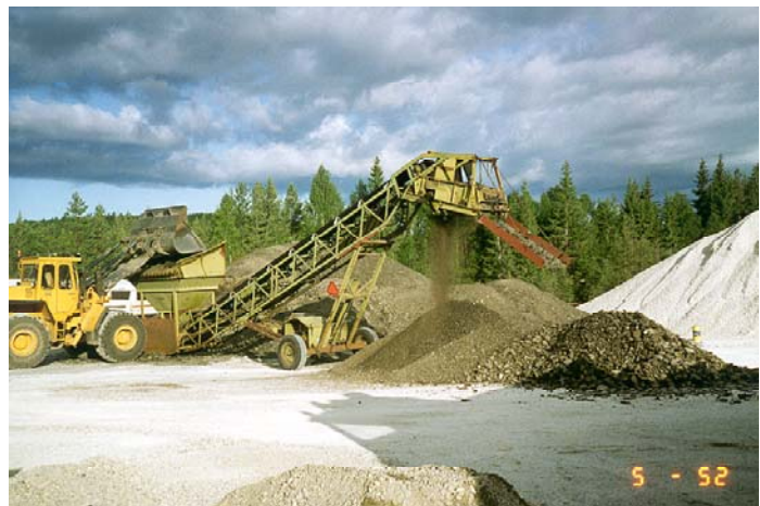
Figure 5 Rough sorting of asphalt granulate. Lumps larger than 22mm should be removed.
