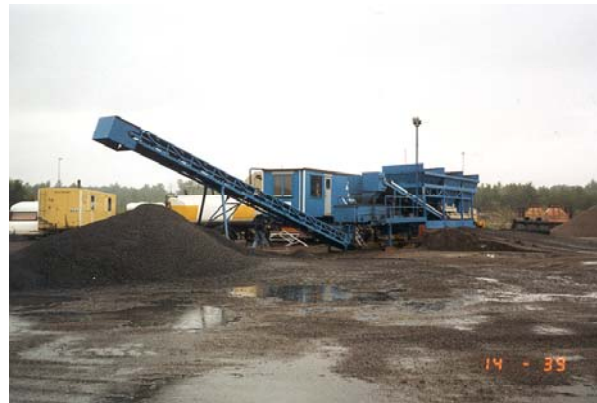
Figure 2 Plant for continuous production of cold recycled mix.
