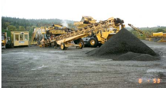
Figure 3 Plant for continuous production of cold mix.
